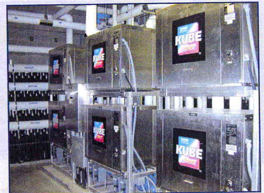
Six or eight Ice Kube units make ice in average full size hockey arena year round. Equipment is easily serviced by local refrigeration mechanics using “off-the-shelf” components supplied by local refrigeration equipment distributors.
